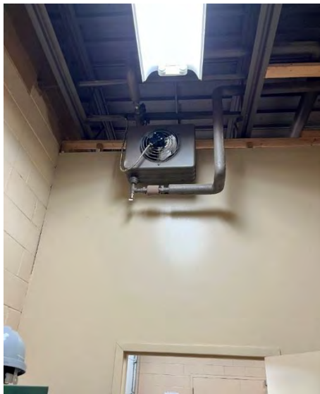
Figure 14 Unit heater outside mechanical room
