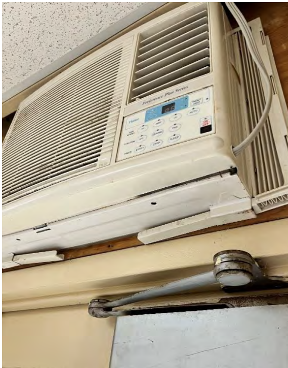
Figure 18 North office air conditioning unit
