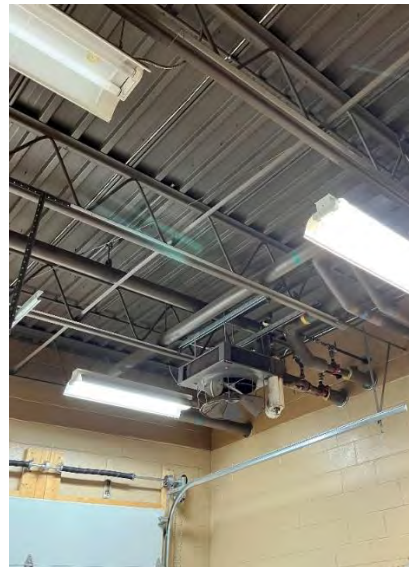
Figure 15 Unit heater in work area
