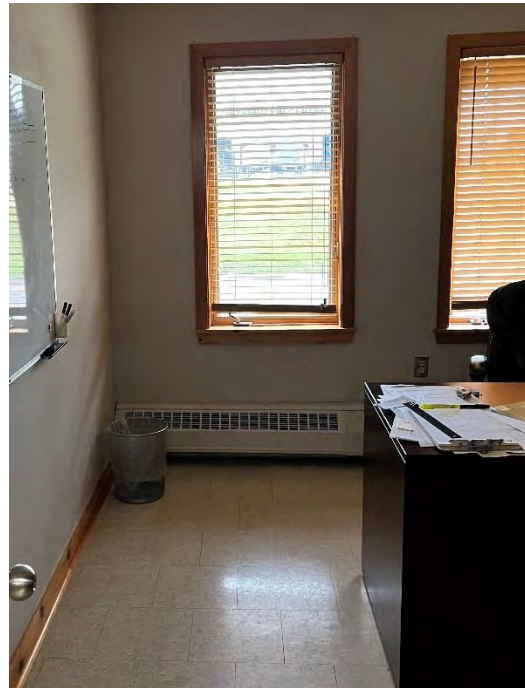
Figure 13 Baseboard heater in north office
