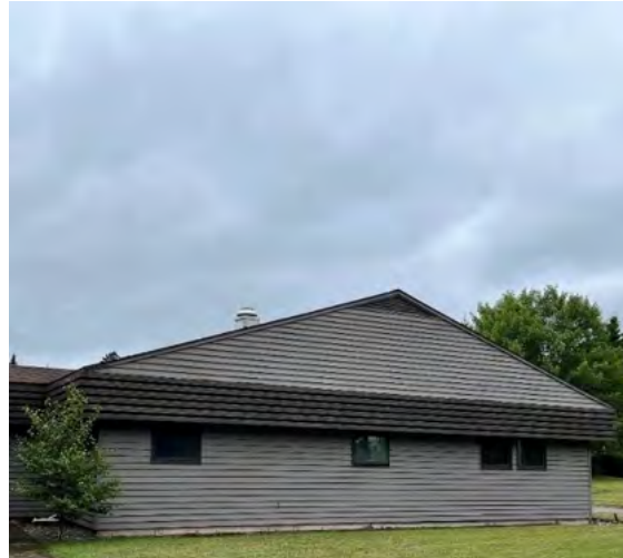
Figure 21 Bathroom exhaust outlet
