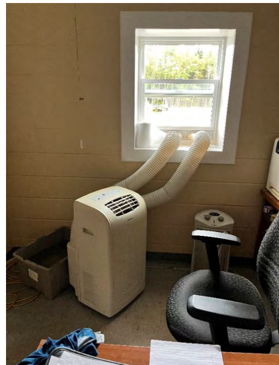
Figure 19 South office air conditioning unit
