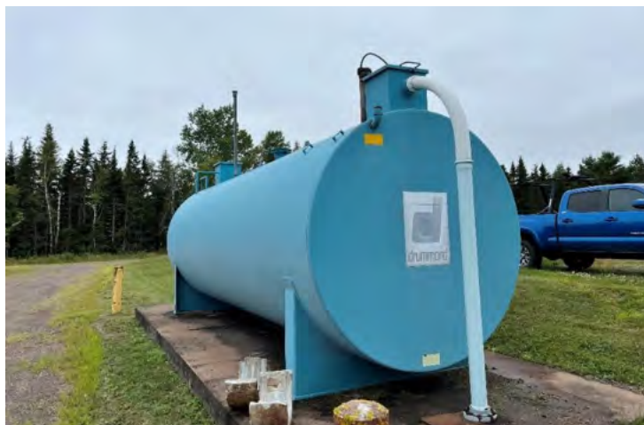
Figure 11 On-site oil storage tank
