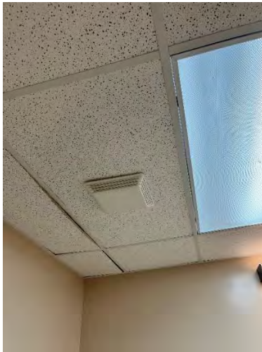
Figure 20 Bathroom exhaust inlet
