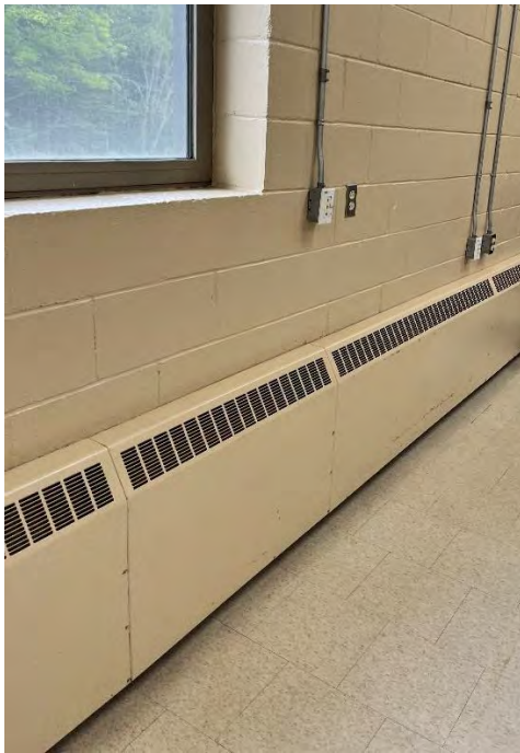
Figure 12 Baseboard heater in meeting room
