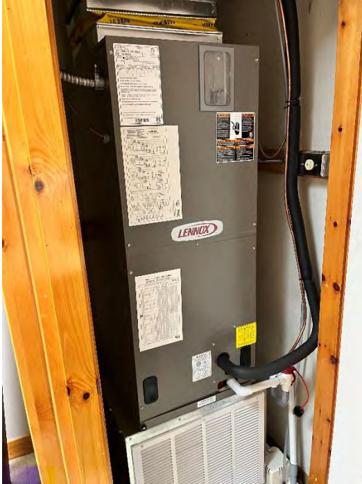
Figure 16 Indoor heat pump unit
