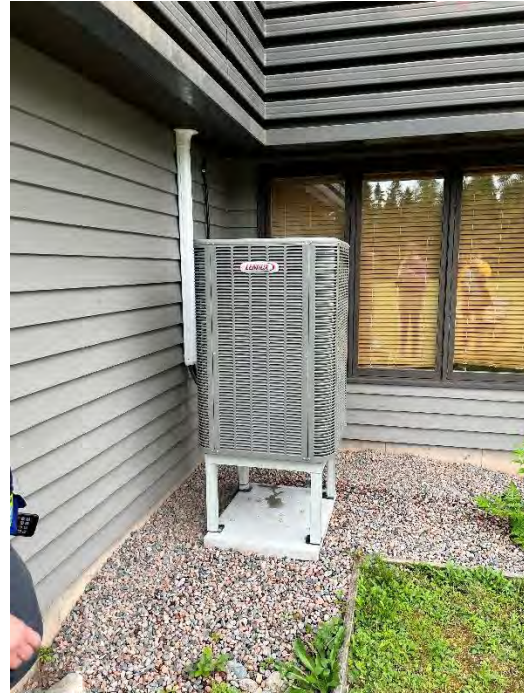
Figure 17 Outdoor heat pump unit
